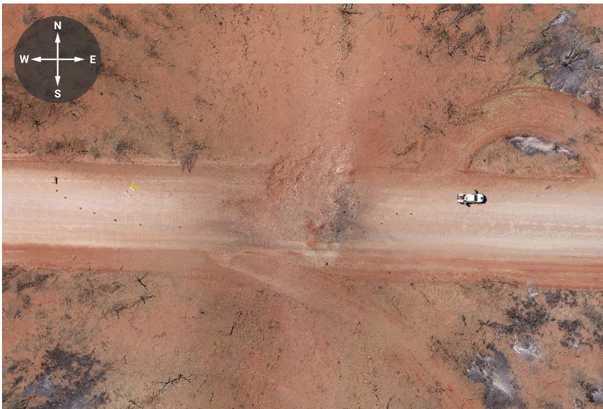
Aerial drone image capturing the crater and the spray of rocks from the road, most pronounced, to the north of the crater (Credit: Gold Fields, Gruyere JV)
