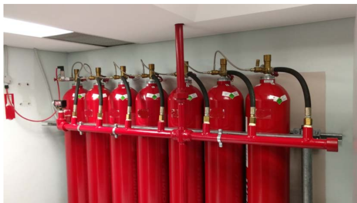
A fire-suppression system's gas storage cylinders.
