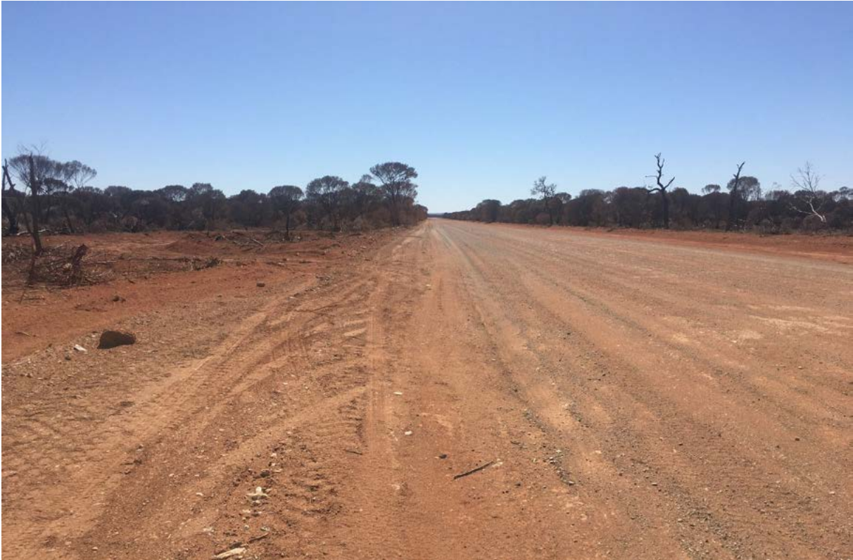
Figure 5.2 Photo of the road looking east (post backfilling of the crater) from the epicentre where it is slightly uphill
