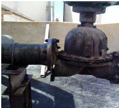
Valve damaged during third acid spill
