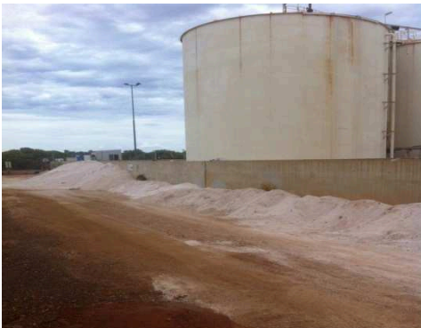
Limestone (piles of pale material) was used to neutralise the second acid spill and support the bund walls
