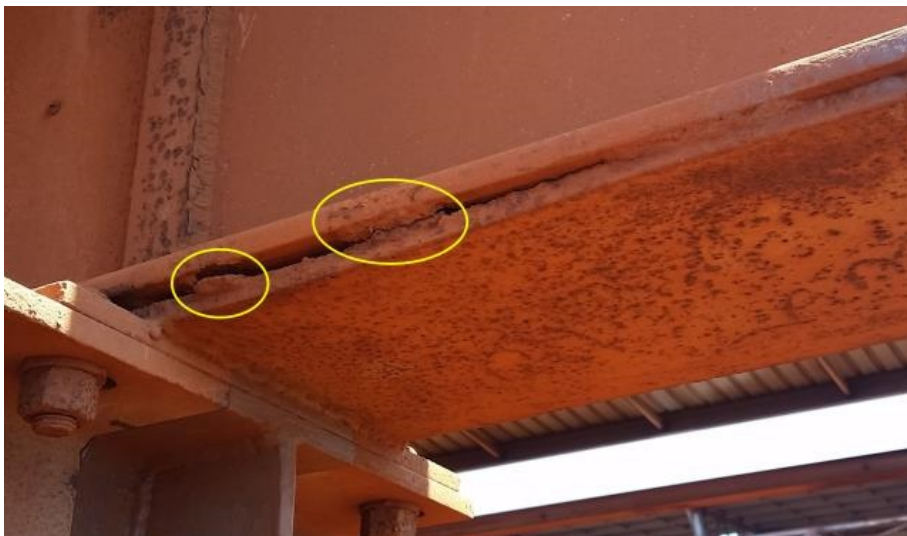
Cracks in site welds after the crane runway was upgraded and structural repairs undertaken.
