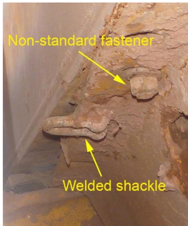
View from below showing non-OEM modifications to the right-hand side of the belly plate.
