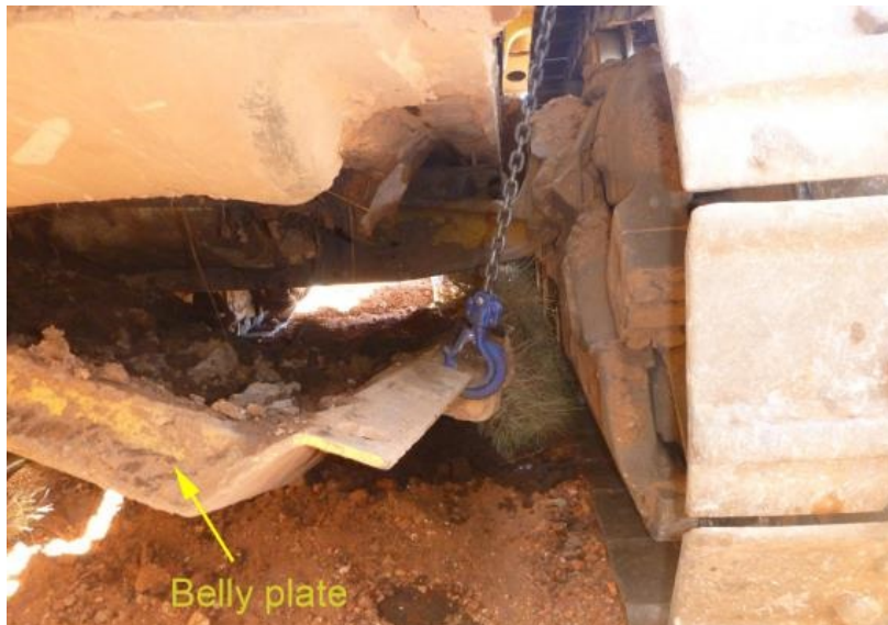
The underneath of the bulldozer showing the belly plate. Note: The come-a-long device has been moved from its position at the time of the accident.
