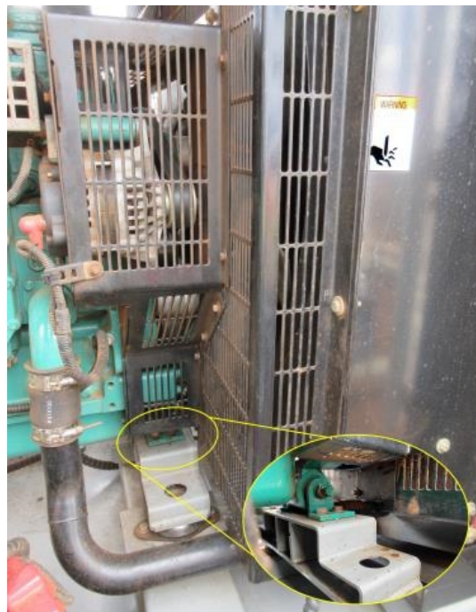
Main photo and inset showing gap in the underside of the guarding as possible access point.
