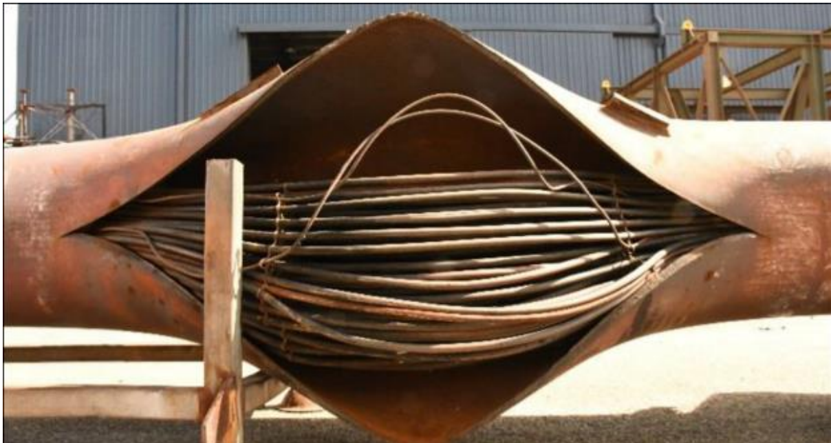
Regeneration gas heater showing area of ductile failure, vessel and heating bundle deformation.
